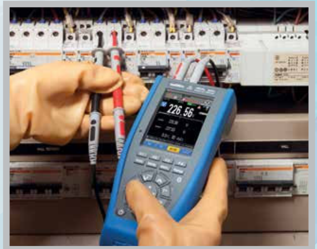
Measurements on electrical cabinets
