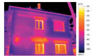
Thermal image with ScaleAssist
